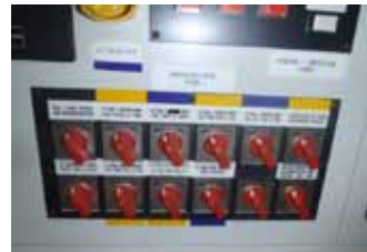
Emergency Stop Panel in ECR
