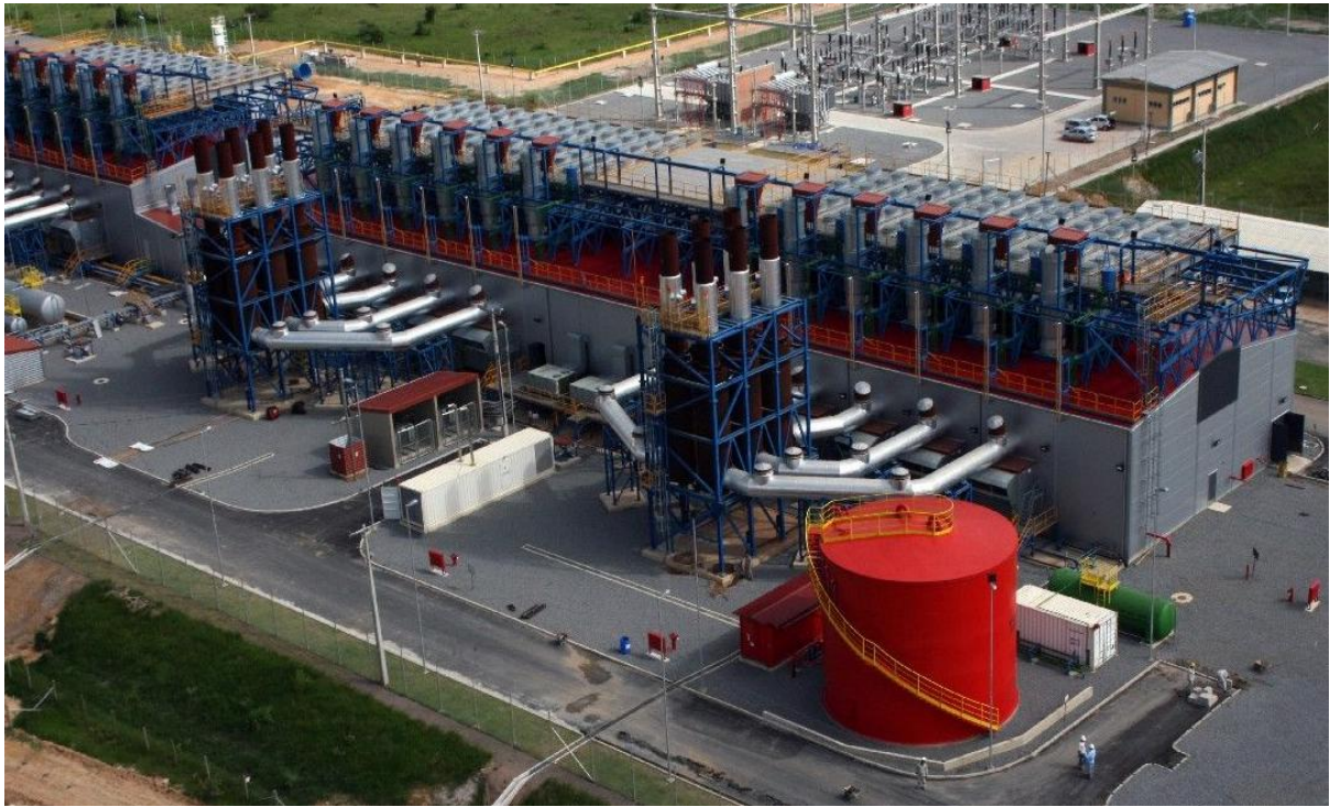
Figure 11. Radiators on the roof in a power plant, Brazil.
