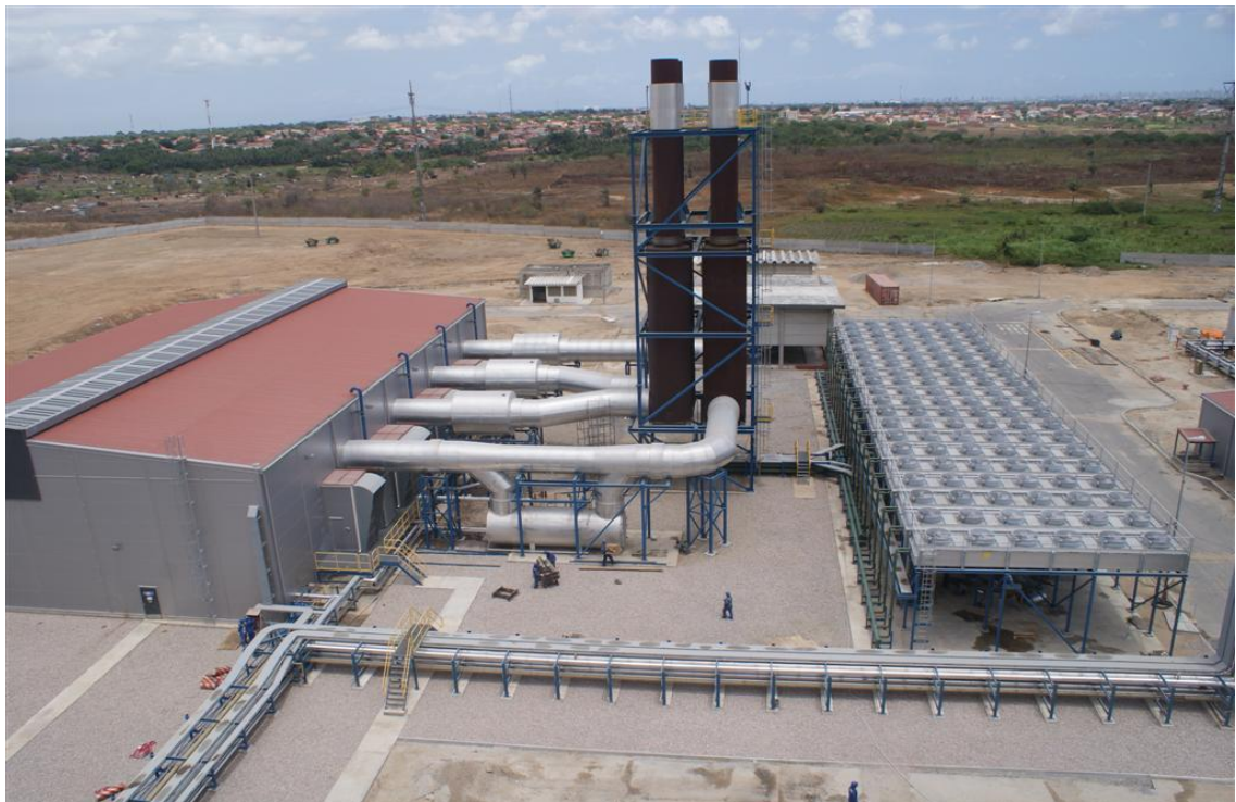
Figure 10. Radiator field in a power plant, Brazil.
