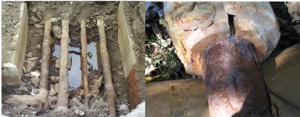
Picture 8. Example of some district heating pipelines condition. /8, p. 35/.
