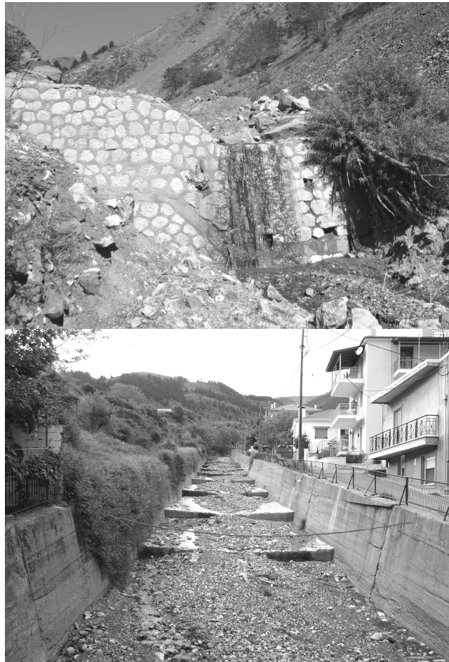
Fig. 1a & 1b - Works for the settlement of the torrent Klarotos. Stone dam for the settlement of branch Kotronakia (1a). Picture 1a shows the extra elevation of the dam in order to make it more efficient. Artificial sheeting of the bed of the torrent Klarotos in the town of Karpenisi (1b). (Source: A. Mertzanis)
