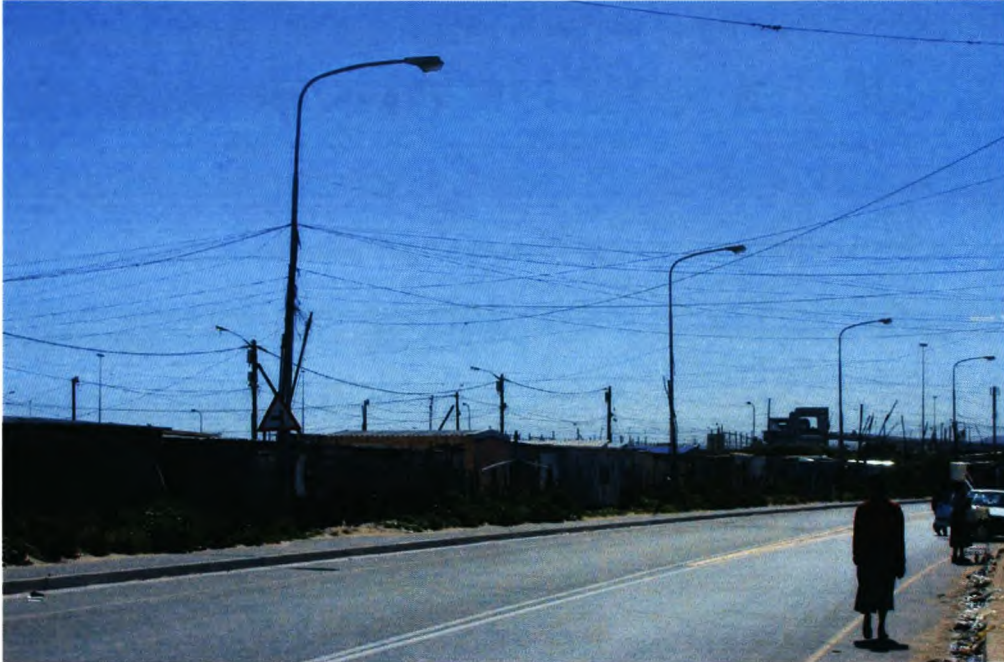
Figure 1.1: An example of illegal connections to the electricity grid.
