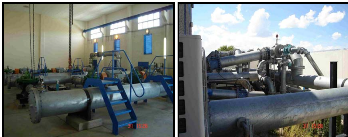
Figure. 7 and 8: The New Western Pump station in Windhoek
