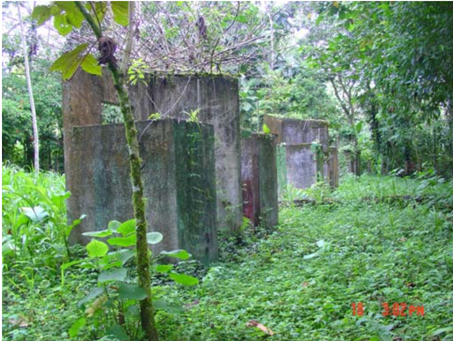
Figure 40. Abandoned picnic area restrooms in La Selva.
