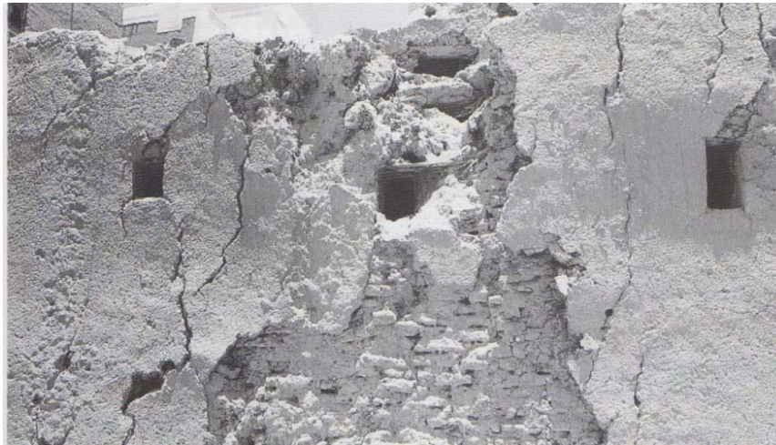
Figure 95. The result of seismic shock and settlement on an earthen structure. Photograph from Conservation of Earth Structures by John Warren, page 187.
