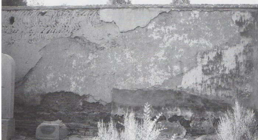
Figure 91. The effect of rising damp. Either there was never a damp course or the damp course failed. Photograph from Conservation of Earth Structures by John Warren, page 147.
