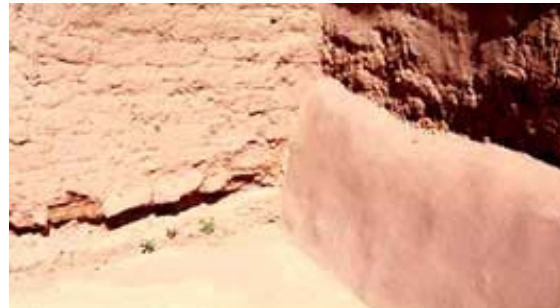
Figure 92. Coving at the base of an adobe wall. Photograph from "Preservation Brief 5: Preservation of Historic Adobe Buildings." Photograph from NPS files.
