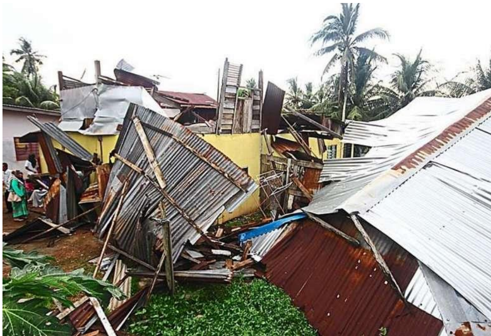
Figure 1.1: Damages caused by the tornado in Kampung Sungai Nonang Source: The Star Online, 13th November 2014
