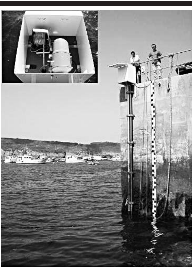
Figure 4. BM 70A radar sensor installed inside a stainless steel tube of 9 cm diameter. The adjoining PVC tube is used to make the probe readings.
