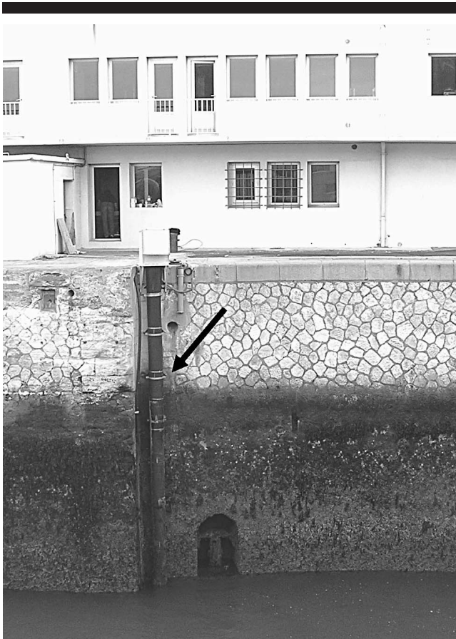
Figure 2. BM 70A radar sensor installed inside a PVC tube of 30 cm diameter, and fixed to the pier with metallic rings (black arrow).
