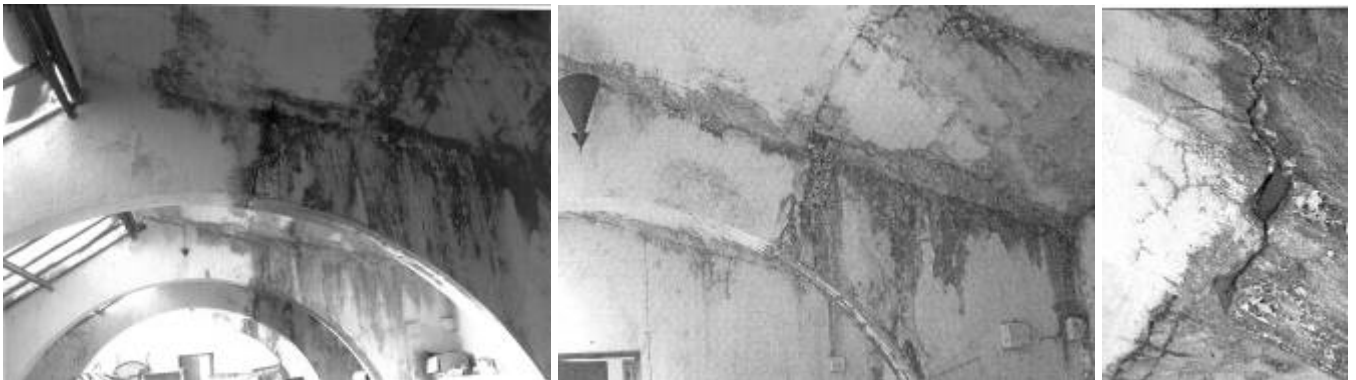
Figure 8. Damages observed on the arches: first or easternmost arch (left), last or westernmost arch (middle), detail of the main crack in the first arch (right).
