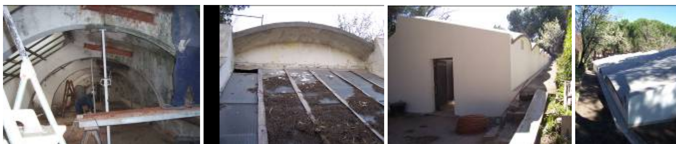
Figure 14: Different stages of repairing and cleaning of the building and the surrounding area.
