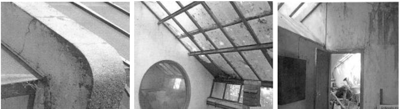
Figure 10. Other damages: main arches, window structure, interior of the east end
