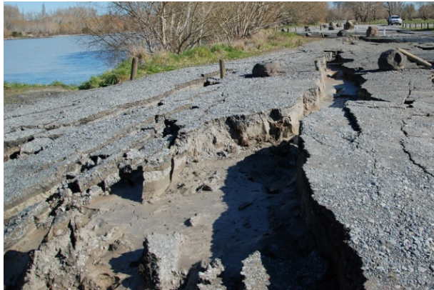
Figure 19 Lateral spreading beside a Christchurch river
