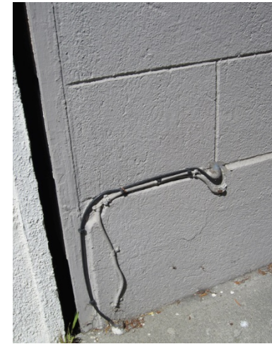
Figure 6 Disguised infrastructure cables of the Marina District
