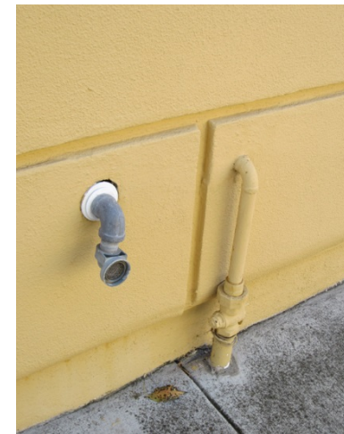
Figure 7 Disguised infrastructure pipes of the Marina District
