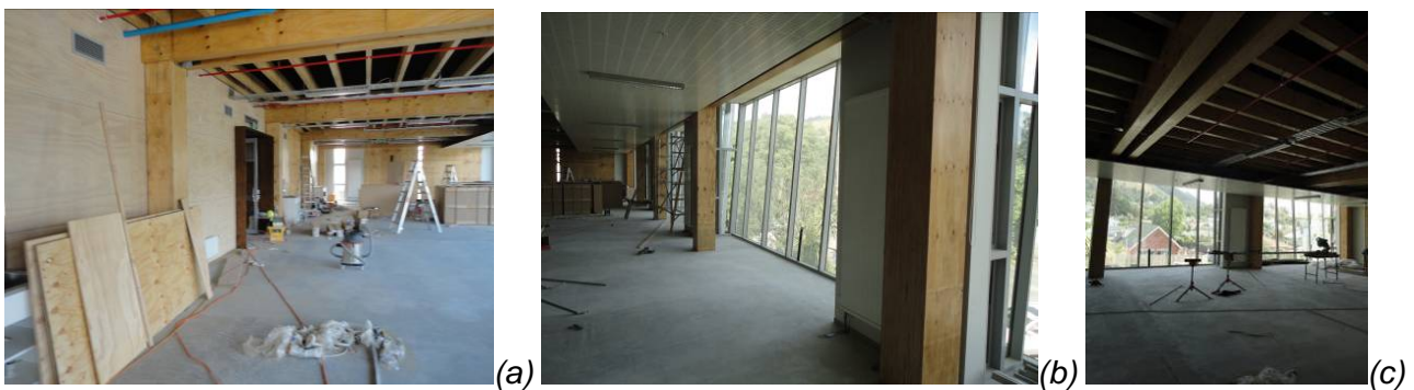
Figure 8-2: Level 2 Studio room 201 (under construction) – Picture (a) internal partition at the north side of the room, picture (b) external wall facing south, and picture (c) room's total transverse span.
