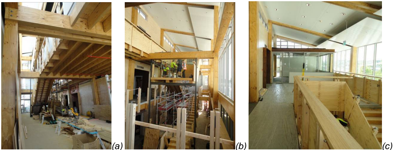
Figure 8-1: Gallery (under construction) – Picture (a) Gallery's Level 1, picture (b) Gallery's Level 2, and picture (c) Gallery's Level 3.
