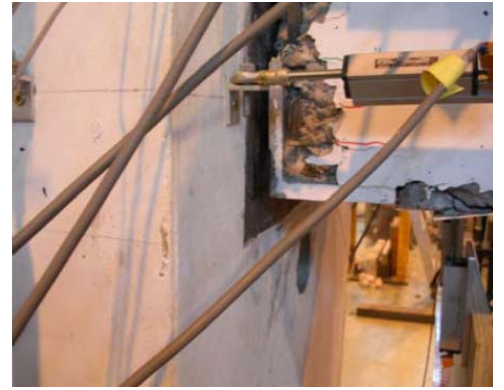
(c) Cover spalling at gravity beam connection
