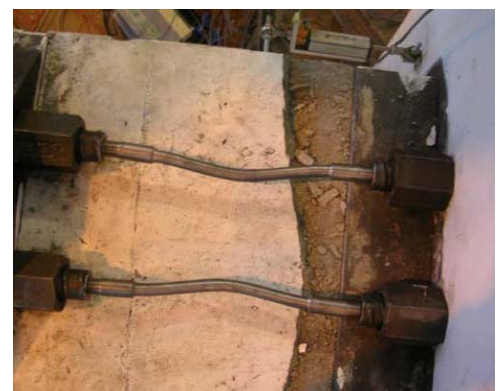
(i) Top view of buckled dissipators after re-centering
