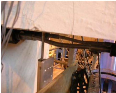
(g) Buckled gravity beam dissipators
