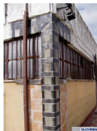
Figure 10. In situ FRP-retrofit of the exterior face of a corner beam-column joint
