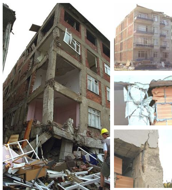
Figure 2. Observed global and local damage in under-designed existing R.C. frame buildings with infills (left and top right, Izmit-Kocaeli and Athens earthquakes in 1999, from NISEE Image Collection; centre and bottom right: Molise event 2002).
