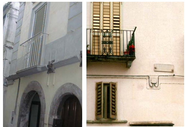
Figure 22. -Top left: Seismic resisting solutions for masonry buildings used in the XIX century and performing well under the June 29, 1873 Belluno earthquake. Use of wooden rafters and beam passing through the full thickness of the walls and well anchored at the edge.
