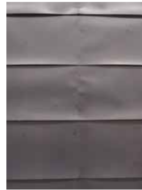
FIGURE 6.95 Cladding with Tetra Pak material
