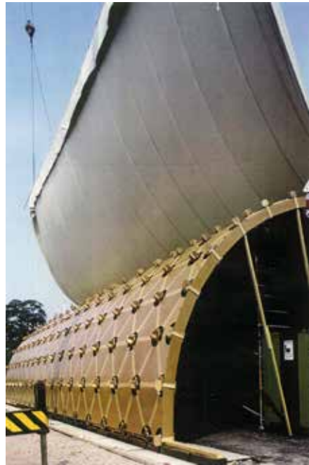
FIGURE 4.25 Watertight membrane covering the cardboard structure with a separate canvas membrane from the top downwards, 1992
