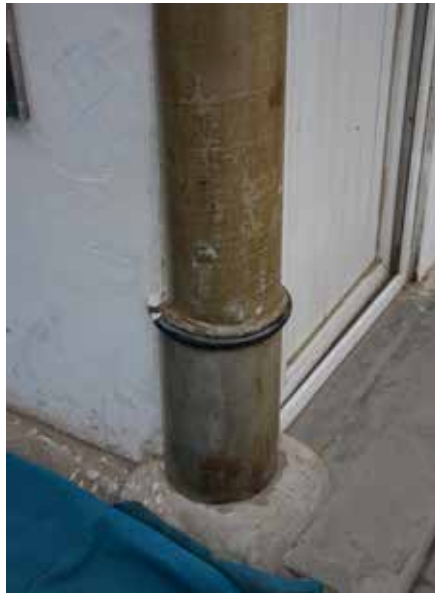
FIGURE 4.81 Hualin Primary School – damaged paper tubes, 2013
