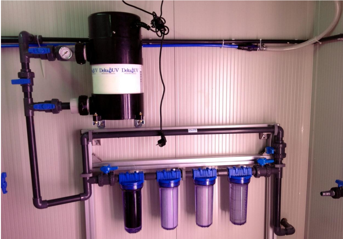
Figure 16 - Sea water treatment composed by filters (60 \mu\text{m} , 10 \mu\text{m} , 1 \mu\text{m} filters), activated carbon; UV light sterilization.
