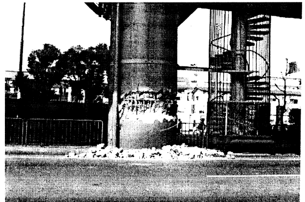
Photo 2 Complex failure mode by tensile and compressive forces
