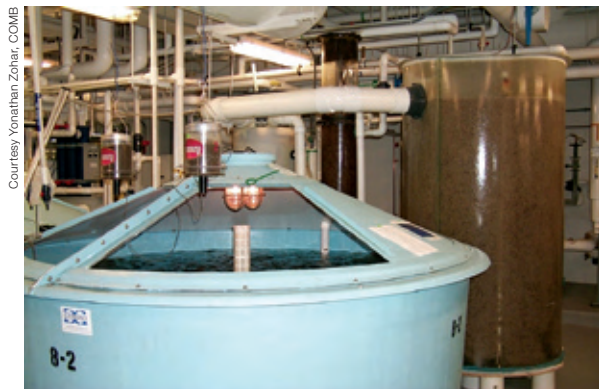
Figure 15. Recirculated fish tank with biofilter (drum on right), which uses beneficial microorganisms to remove chemical wastes from the water
