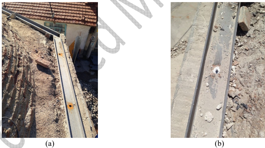
Fig. 7. Steel girder elements at the top of the drum, (a) single U160 elements, (b) steel anchor connection
