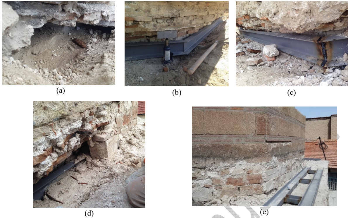
Fig. 6. Implementation of the steel girders at the bottom level of the drum, (a) loss of wooden beams, (b) steel girder elements placed at the bottom section of the drum, (c) welded connection of steel girder elements, (d) hydraulic lime-based injection and covering, (e) covering the elements with new masonry material
