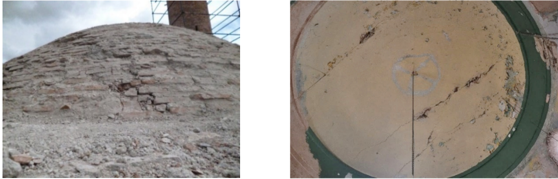
Fig. 4. Large cracks observed on the dome exterior and interior
