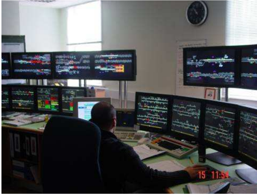
Figure C- 20: IECC Signal Box
