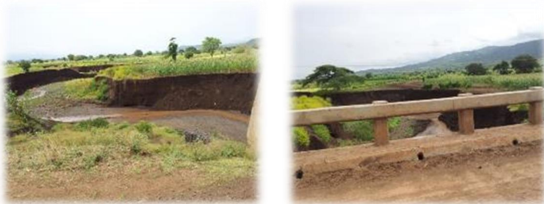
Figure 56: Poor road construction opening-up huge gully water ways to Lake Chamo
