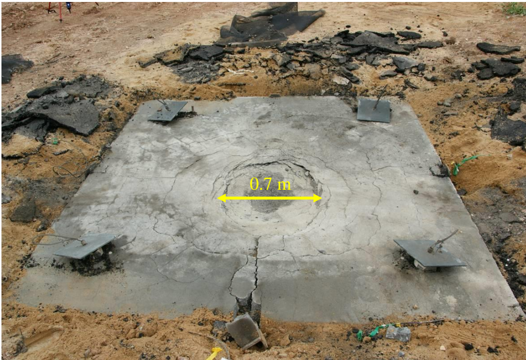
Figure 20. Damage of proposed multi-layer pavement after blast (after removing AC layer)
