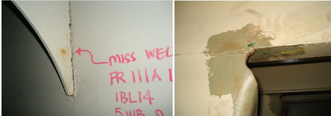
Fig. 10: Defects on a vessel are marked directly by the surveyor
