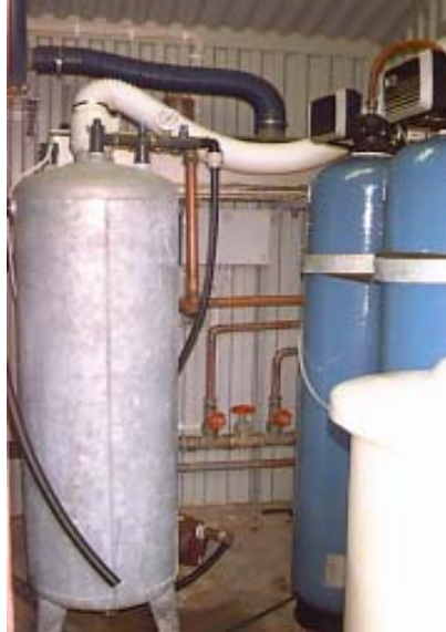
Figure 4. The Radonfällan aerator (left) and the two cation exchangers (right) in the Grinduga waterworks in Furuviik.
