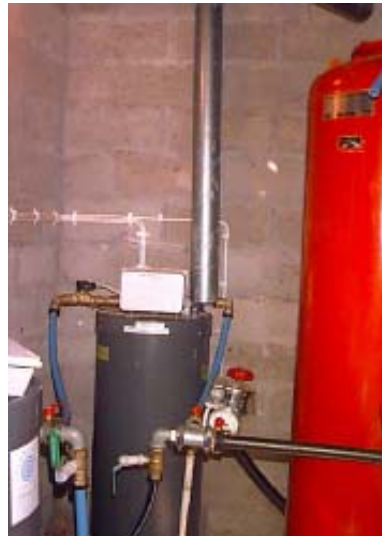
Figure 7. Two Libradon aerators (on the left) are utilised for radon removal in the Kråkbodarna waterworks in Leksand. A pressure tank is located on the right.
