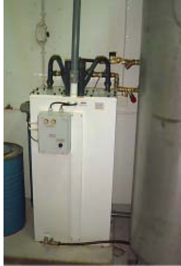
Figure 6. The Radonett aerator is applied for radon removal in the Sjugare waterworks in Leksand.
