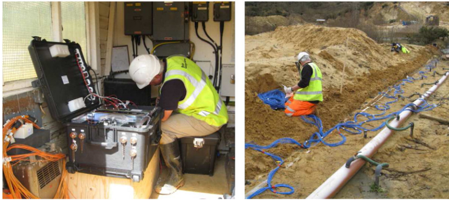
Fig. 2. ALERT instrument installation (left). Electrode monitoring array installation (right) – the well-point groundwater extraction system can be seen running parallel to the electrode array.
