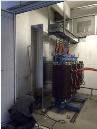
Fig. 1 Local shield for the power transformer
