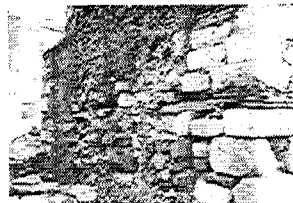
Figure 3. View from the north wall illustrating structural and material problems.
