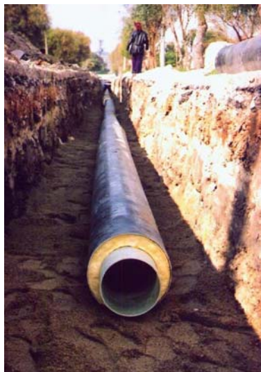
Figure 3.4 Fiberglass pipe (composite) that is used in Çeşme Geothermal District Heating System.
