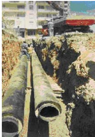
Figure 3.3 Carbon steel pipe that is used in Balçova Geothermal District Heating System in Izmir [37].
