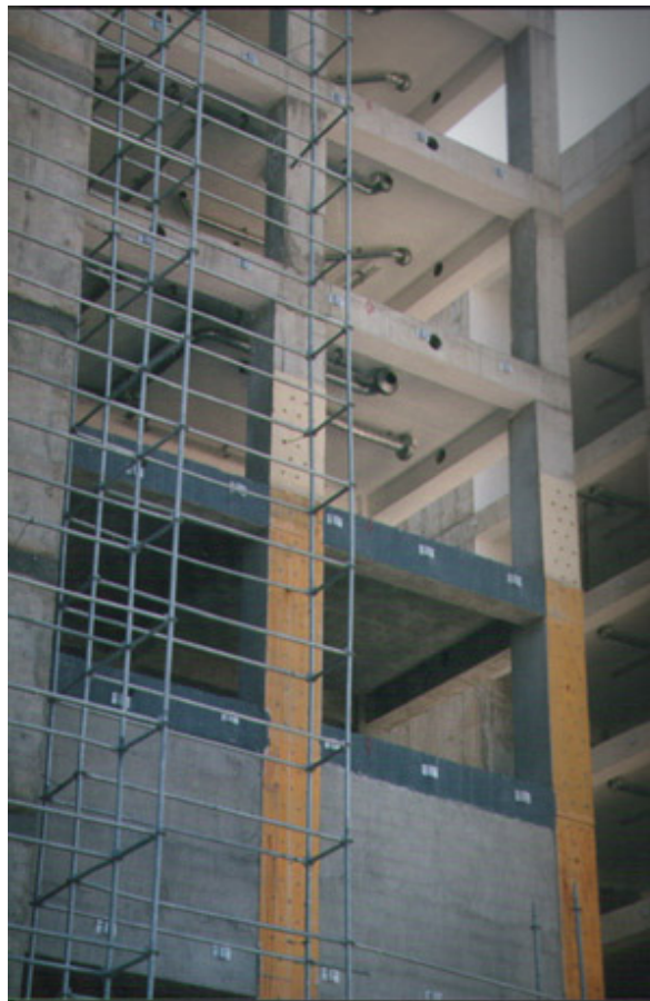
Fig. 4.22. VRV/HRV System Channels Cut Through the Beams
