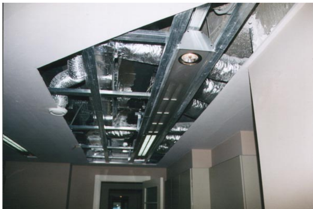
Fig. 4.6. Installations, Pipes and Lighting Channels Hidden in the Suspended Ceiling
