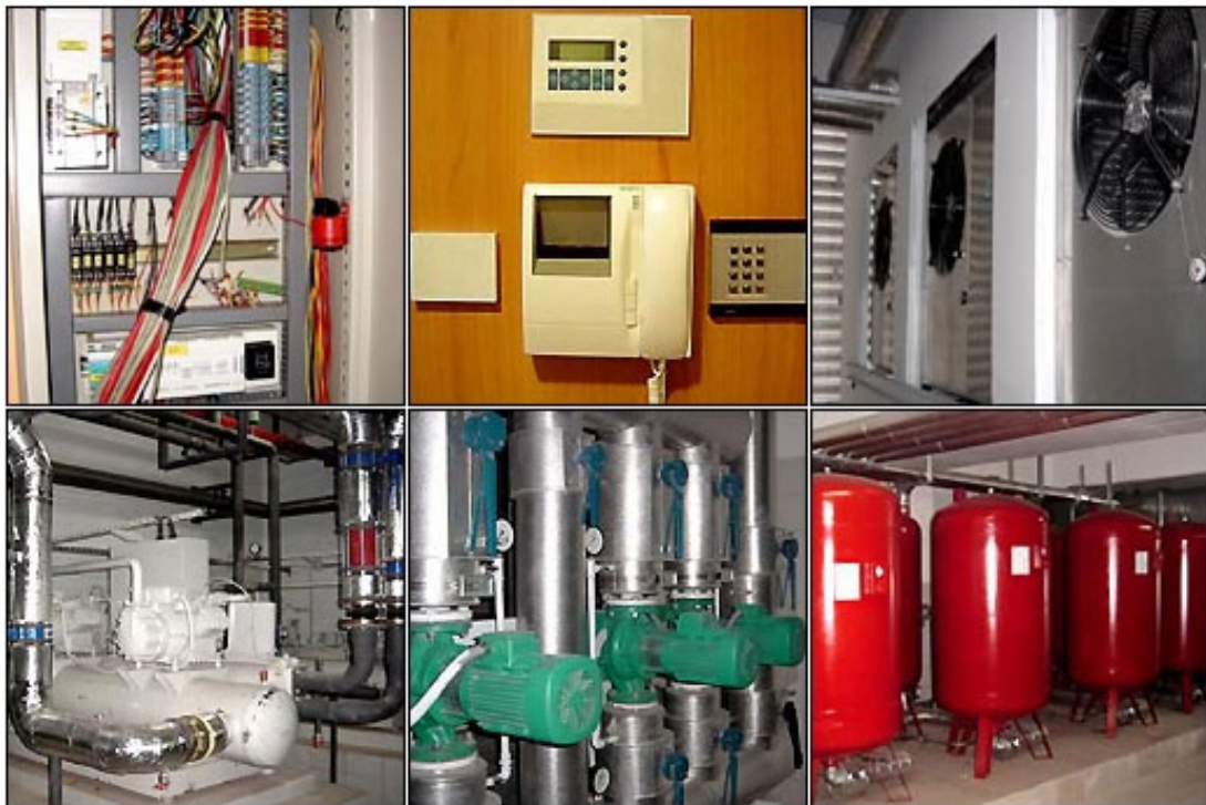
Fig. 4.10. The Indoor and Outdoor Panels, Chiller, Water, Heating and Fire Systems of Polat Tower (Source: http://www.polatinsaat.com )
