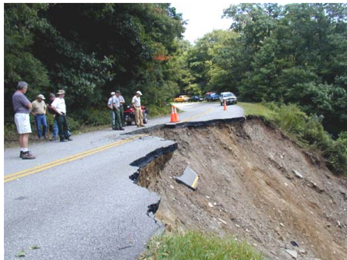
Figure 2.12. Blue Ridge Parkway (Milepost 348) fill-slope failure that initiated Bear Drive Branch National Forest, North Carolina debris flow on Pisgah (Source: Hurricane Frances, September 2004)
