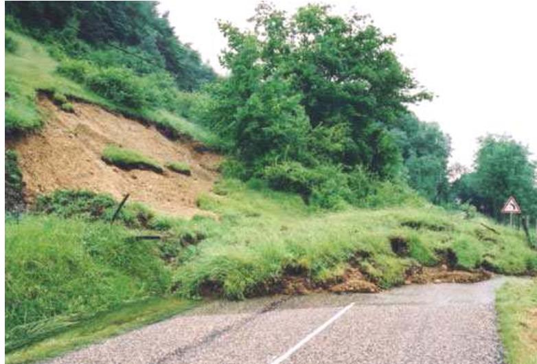
Figure 3.1. Shallow Landslide in Merlas-Isère, South-Eastern France
