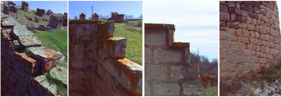
Figure 20. Material deteriorations and unqualified repairs in the towers in the masonry walls.
