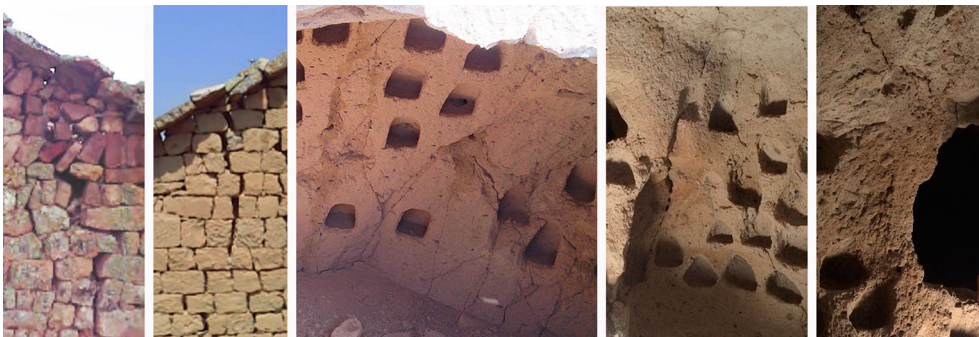
Figure 19. Structural failures: Cracks in the walls of the towers and cracks in the walls of the nests and superficial erosion in the rocks.
