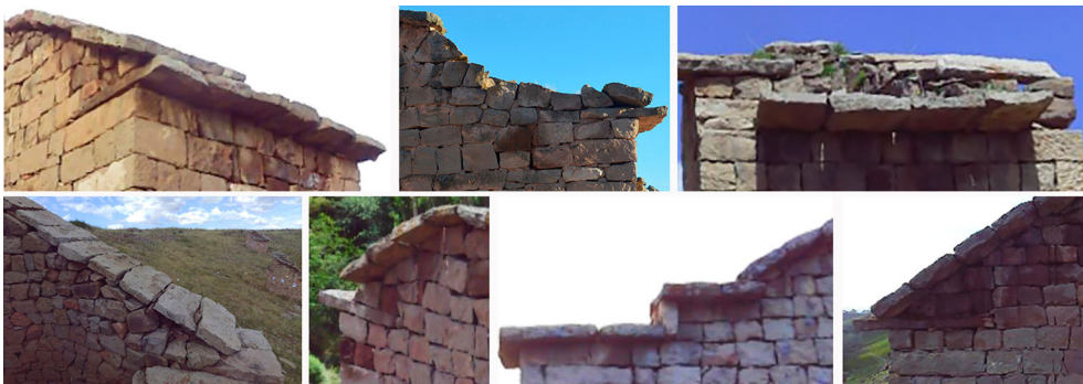
Figure 16. Eaves in the dovetails built with rough-cut stone masonry: different applications and special details.
