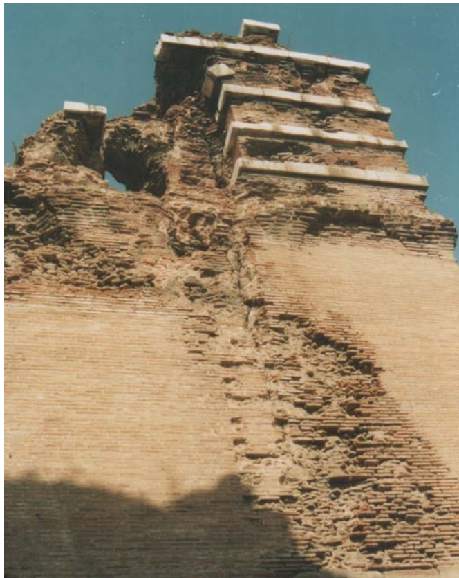
Figure 4. 98. Loss of material in the south-west elevation (2004)
