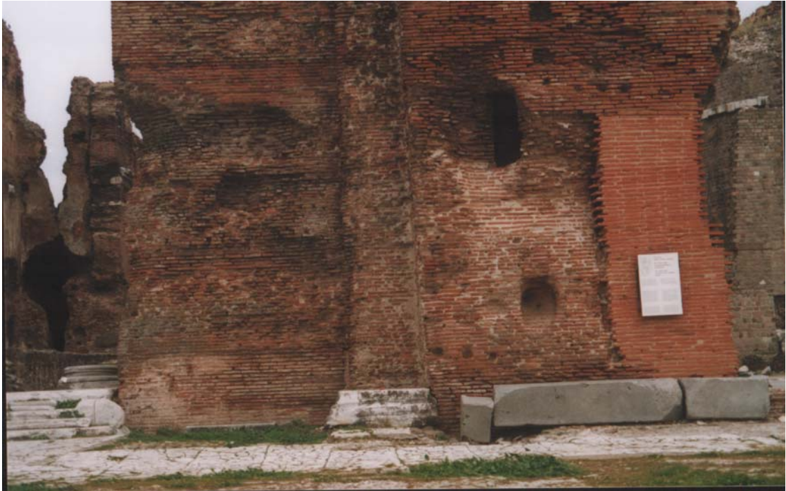
Figure 4. 95. The building materials is affected by soluble salts (2004)
