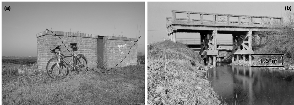
Fig. 2 – Evidence of the anthropogenic land subsidence in the reclaimed area: (a) The protrusion of a sluce well above the bed of an old disappeared channel; (b) An old bridge hanging over the canal bank which settled by 1.5 m.
