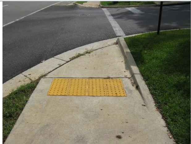
This is another bad example of an incomplete detectable warning.
