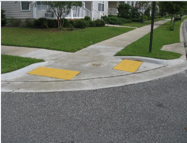
This is an bad example of an incomplete detectable warning.
