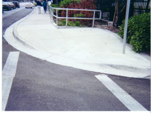
This is another bad example of a missing detectable warning.
