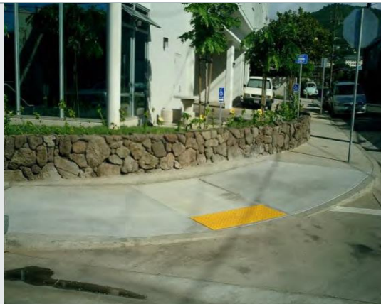
This is an example of a good parallel ramp.
