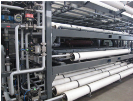
Photo 1. A Reverse Osmosis (RO) installation.
