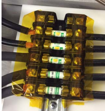
Fig. 10 Fuse block insulation.
