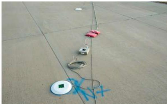
Figure 5. NeAR module installation at Edwards. The microphone is on the round plate. The NeAR module is the square box.
