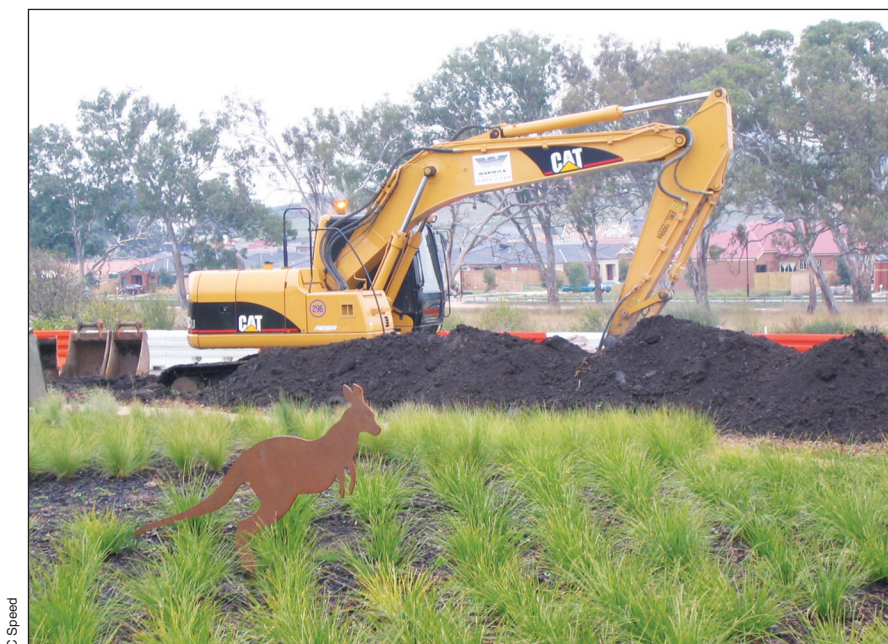
Figure 3. A residential development site in northern Melbourne, Australia, whereby impacts to the grassland ecosystem were offset elsewhere. Installations of metal wildlife-themed statues as part of an interpretive walk only serve to highlight the loss of biodiversity from the area.
