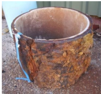
Figure 1 Example of general corrosion in cast iron water mains [8]
