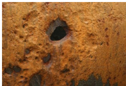
Figure 3 Example of pitting corrosion in cast iron water mains [8]
