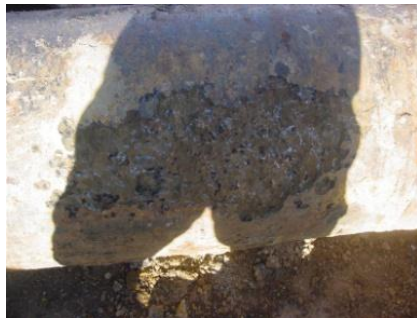
Figure 2 Example of patch corrosion in cast iron water mains [8]
