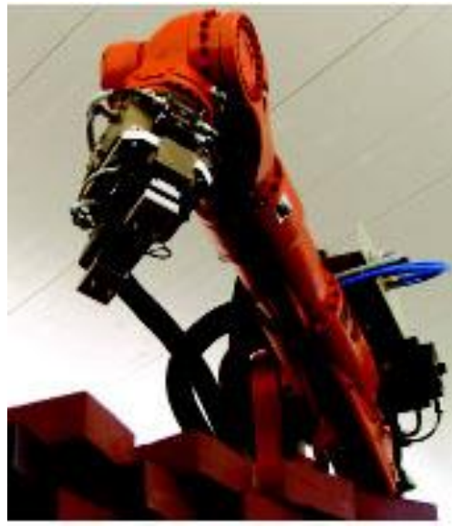
Figure 14. Construction of a brick wall by a robot hand, Tobias Bonwetsch, Daniel Kobel, Fabio Gramazio and Matthias Kohler, Zurich, 2006. 167
