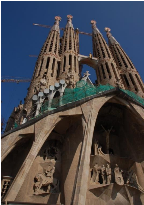
Figure 58. Full scale mock-up of finials tested on the Passion Façade at the construction site of the Sagrada Família , Barcelona, 2008. 468
