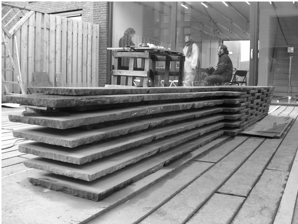
Figure 66. Scenes from the construction of the slate wall: Top photo showing Hayim Beraha (on the left) and Sinan Ilhan constructing the wall, bottom photo showing (from left to right) Sebastian Veldhuisen, Ceren Balkir and Hayim Beraha having a break at the background, Ypenburg, The Hague, 2007.
