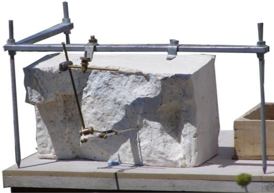
Figure 42. A pantograph used by stonemasons for replicating missing stones at Sagalassos archaeological site, Antalya, Turkey, 2006. 347
