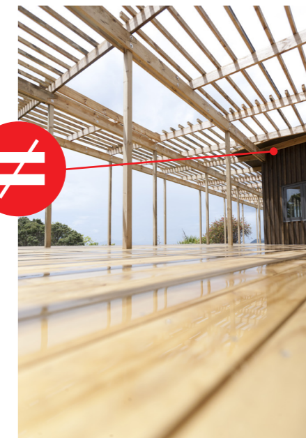
figure 3.5: pergola-to-cladding detail discrepancy at Langs bach photography: Sajeev Ruthramoorthy
