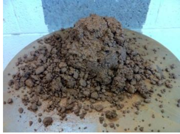
Figure 15 - Material under FMP, showing crumbling.
