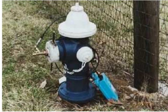
Figure2. Instrument installed at a fire hydrant
