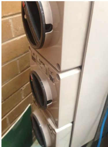
Figure 7-2 Switches for the heating elements
