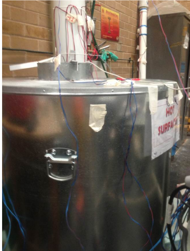
Figure 7-1 Hot water tank
