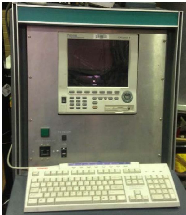
Figure 7-47 Data logger system
