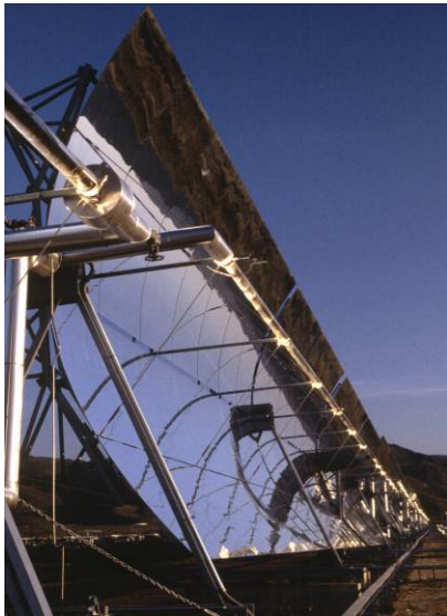
Conc. Solar Collector
