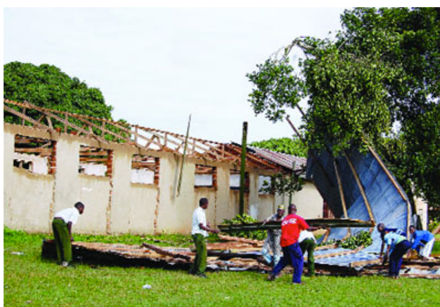
Photo 2: a school building whose roof came off during a classroom session in a rainstorm.
