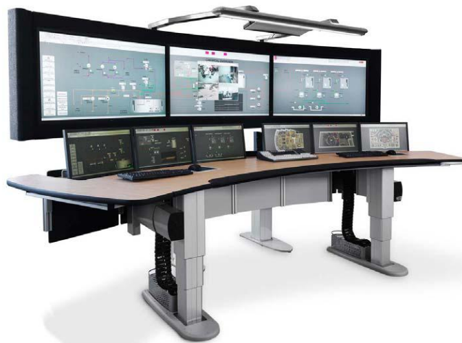
Figure 29: Main CR LSD and Operator stations (Type EOW-x3, delivered by CGM)
