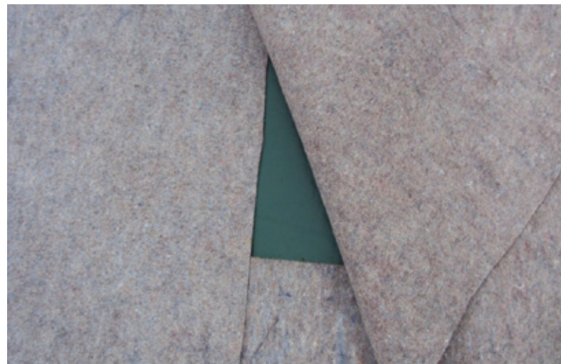
A protection mat is laid to protect the waterproofing layer on a green roof
