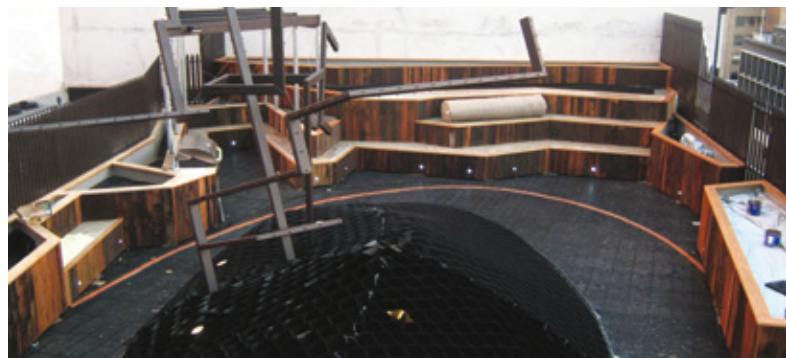
The build up of this green roof 'hill' in Queen Street, Melbourne, is created from recycled expanded polystyrene blocks, overlaid with a deep drainage layer to contain the growing substrate
