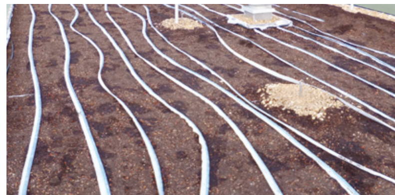
Laying irrigation pipe at Minifie Early Learning Centre green roof. Image: Junglefy
