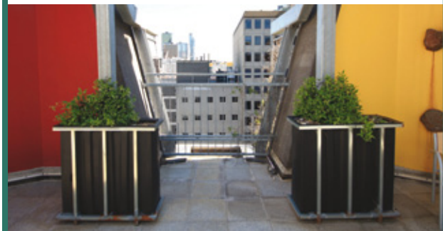
Planter boxes on the City of Melbourne's Council House 2 roof garden, Little Collins Street, Melbourne, have not performed as well as expected
