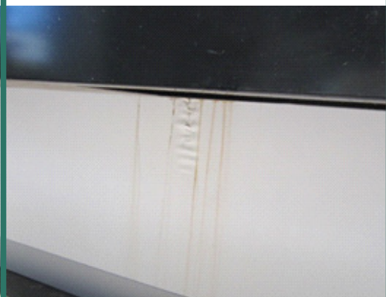
An improperly sealed joint created a leak behind this green wall
