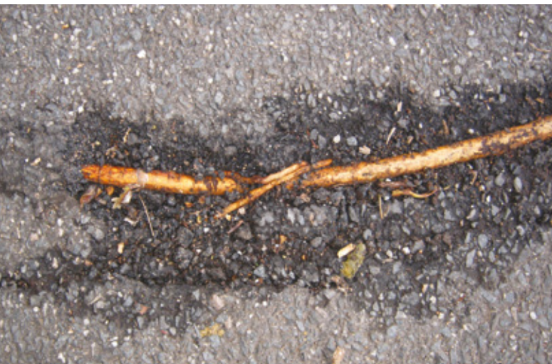
Plant roots can be very destructive, as shown by this image of tree roots causing severe cracks in bitumen paving. A root barrier on a green roof can protect the underlying layers
