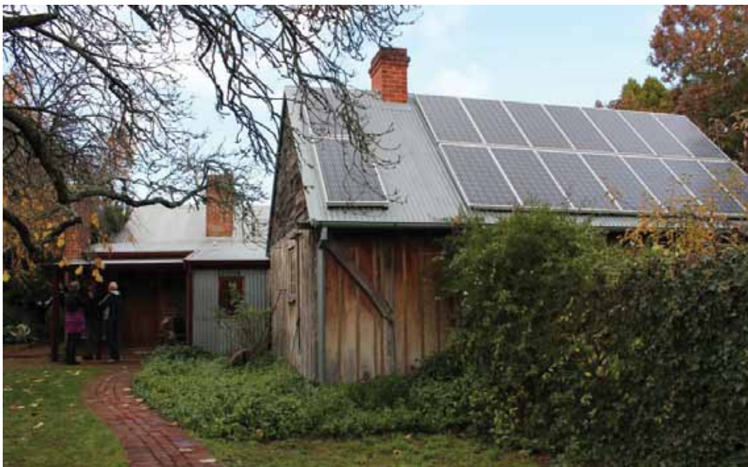
Figure 5: Solar PV on Hahndorf historic house, South Australia
